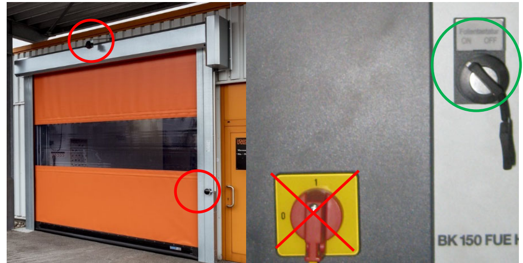
Impulse generator in the outdoor area
