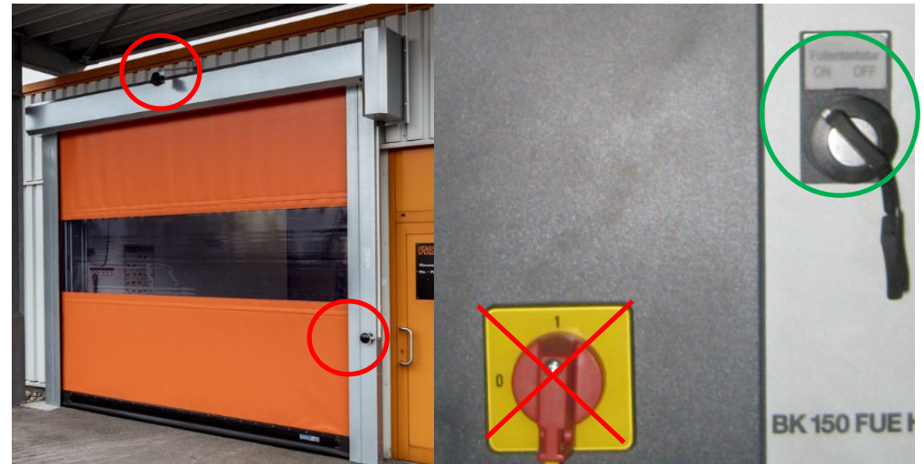
Impulse generator in the outdoor area
